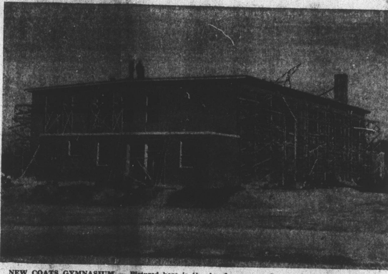
NEW COATS GYMNASIUM — Pictured here is the handsome new Coats school gymnasium, which is nearing completion. The structure, which will cost over $100,000, should be ready for use by early spring and Principal Hal Smith says the basketball team is planning a game in it no matter how late it might be. At present, the team is having to practice outdoors. The gym will fill a vital need in the Coats community. R. M. Turlington of Lillington is the general contractor. (Daily Record photo by T. M. Stewart).
