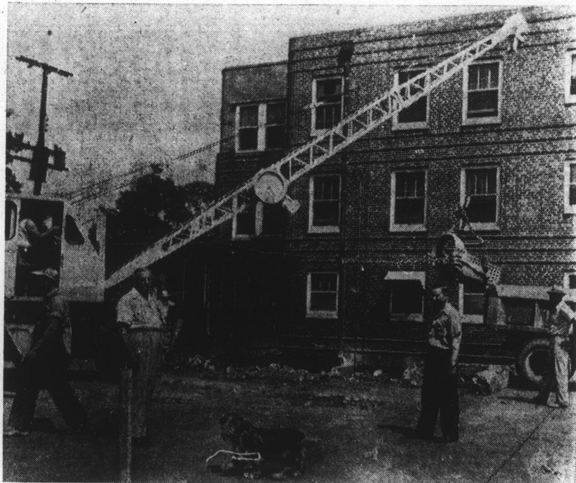
WORK STARTED ON HOSPITAL ADDITION — Workmen have begun construction on the new $100,000 addition to Dunn Hospital, Inc. A big crane is shown here in operation as the excavation got underway. Shown standing in front of the crane is M. E. (Pop) Winston, manager of the hospital, and facing him is N. B. Hudson, one of the hospital aides. Contractor for the project is Rogers Construction Company of Smithfield. (Daily Record Photo by Ed Welborn).
