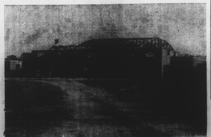
NEW GYMNASIUM NEARS COMPLETION — Shown is the new gymnasium, part of the Campbell College Expansion Program, which is rapidly nearing completion and which should be ready for some basketball games this season. The structure will fill the need for a suitable place for athletic and other events on the campus of the Harnett County institution. Under its expansion program, Campbell College is planning to improve its facilities in order to offer students of the area it serves, the best in Junior College education. (Daily Record photo by T. M. Stewart.)
