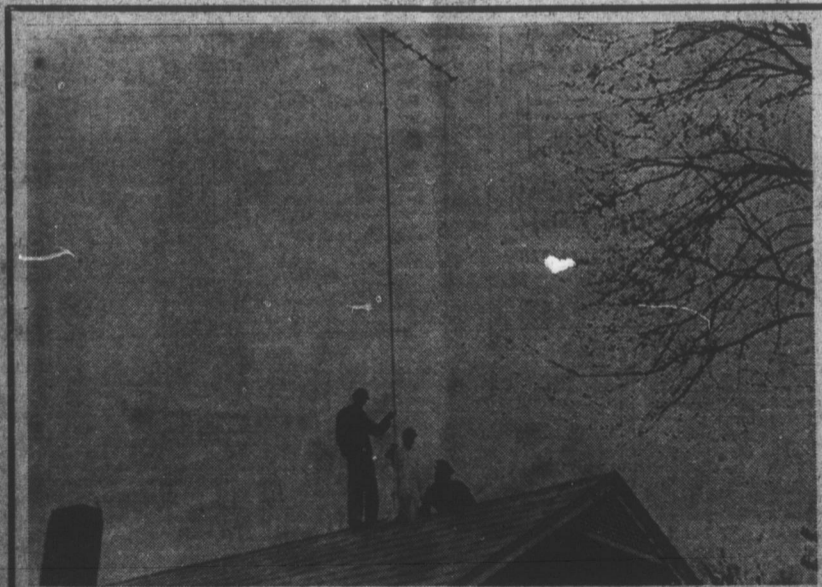
Two of Purdie's expert TV Technicians are shown here installing a television antenna at the home of Mr. and Mrs. R. L. Adcox at 607 S. Fayetteville Ave.
