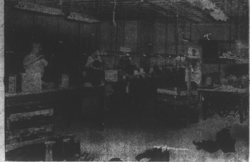
GETTING READY FOR BUSINESS — Harry Fisher and James Bunting, two employees of Benjamin and Johns, sent here from Newark, N. J. are shown setting up the machinery for the new plant which is scheduled to begin operating here on May 1st. The machinery shown is in the store building vacated by Thomas and Warren's furniture store. In addition to the 96 machines in this section, an additional 32 machines will be installed in the adjoining store. The last of the machines should arrive here by April 27. (Daily Record photo by Louis Dearborn).
