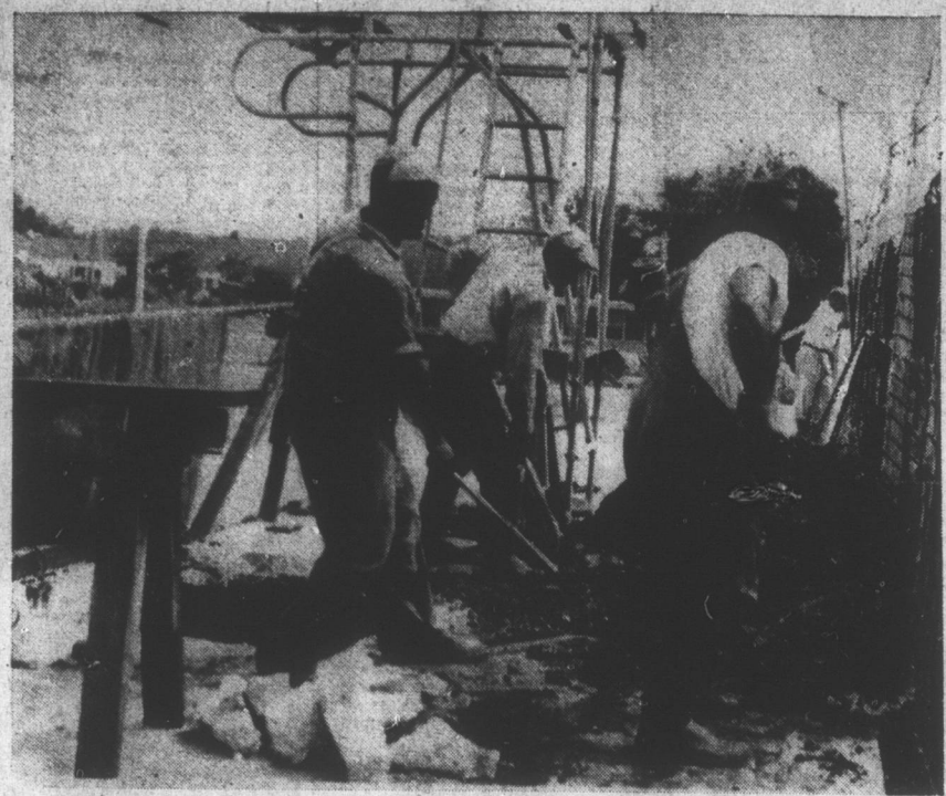
PLUGGING THAT LEAK - Workmen of the Water Department are shown here completing the repairs on the leak in the Dunn Swimming Pool. The town board, at a special meeting held at the pool yesterday, authorized the repairs and no time was lost in getting the job done. The pool was partially drained this morning and a new section of pipe put in. It was refilled and ready for use this afternoon. Every effort was made to avoid any lengthy shutdown of the pool during the present hot weather. (Daily Record photo by Louis Dearborn).
