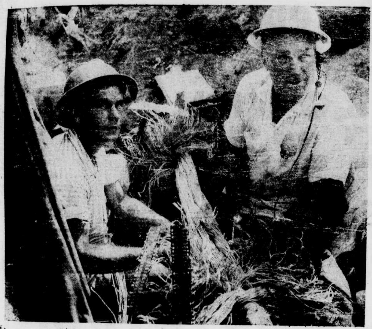
WILD ASSORTMENT of wires have to be carefully paired together as telephone crewmen L. B. Fields (with earphones under his hard hat) and fellow cable repairer E. L. Ovenden (left) struggle to return service to Coats, Erwin area. (Record Photo by Ted Crail.)
