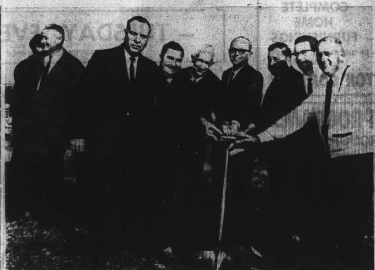
PROJECT GETS UNDERWAY — As County Commissioner Willard Mixa smiles his approval in background, Mayor Bill Marshburn and other city officials are shown here digging the first shovel of dirt to start construction of Dunn's new city hall. Left to right holding the shovel are: Commissioners Bill Godwin, Mayo Smith, City Manager Archie Uzzie, Mayor Marshburn; Commissioners Howard Hardy, Bill Cameron and Paul Perry. (Daily Record Photo by Russell Bassford.)
