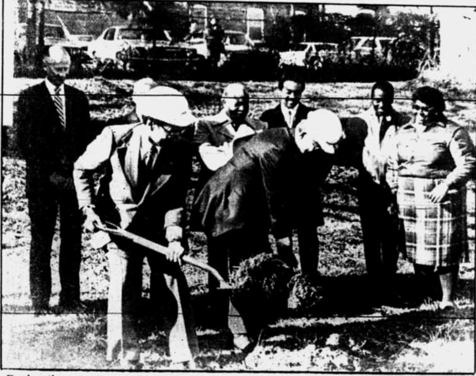
During the recent ground-breaking for a three-story residence hall on the campus of Johnson C. Smith University, Dr. Robert L. Albright (l) and Dr. Mathew J. Whitehead are shown with members of JCSU's Board of Trustees.
