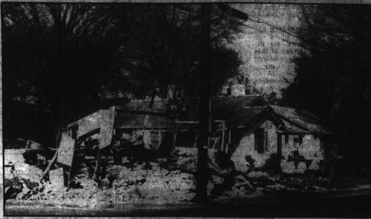
The owner of the dilapidated property located on the corner of Davidson and 18th St. responded to the neighborhood group's request to have the eyesore bulldozed.
