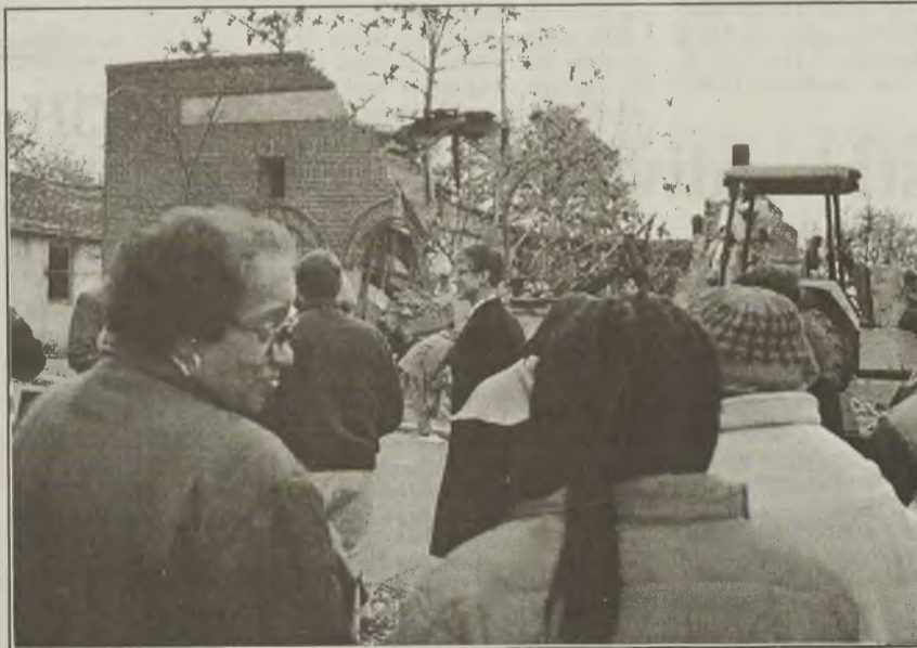
A crowd of 75 looks on as the building, which was once a church, is demolished. The lot will be used for parking for local churches.
