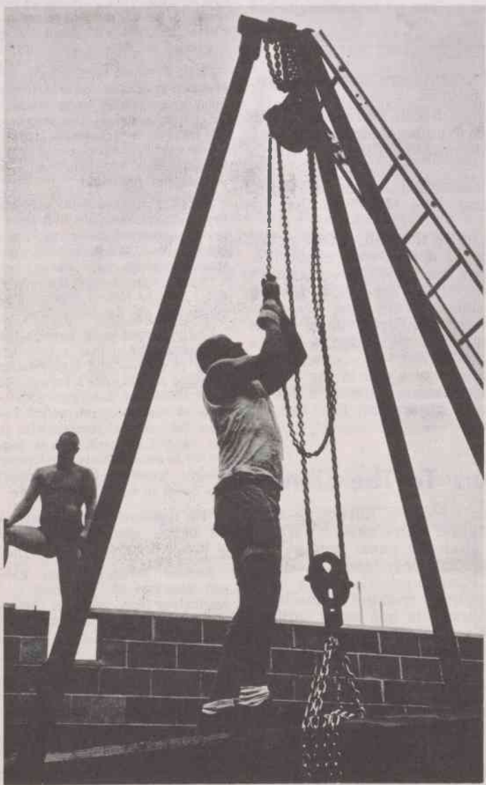
GOING UP! —This photograph, made during construction of the School of Graphic Arts at Chowan College, shows two students on the job. Hoisting part of the framing is Martin Forbes of Norfolk, while Charlie Stephens looks on. Both were summer school students at Chowan and now are attending VPI where they play on the football team.
