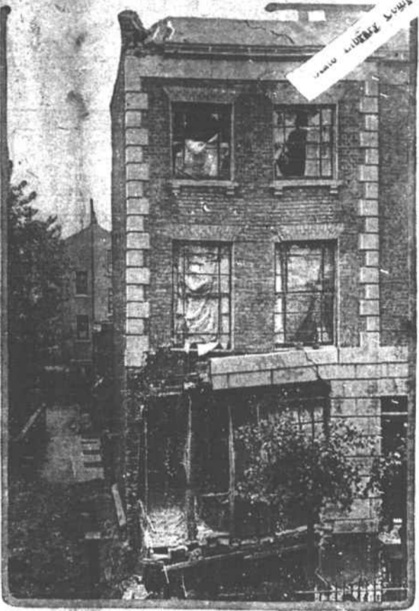
What the bombs dropped from the German Zeppelins in their recent raids over London did to the buildings where they fell is well illustrated by this photograph of a house in Shakespeare road, badly wrecked and seemingly about to collapse.
