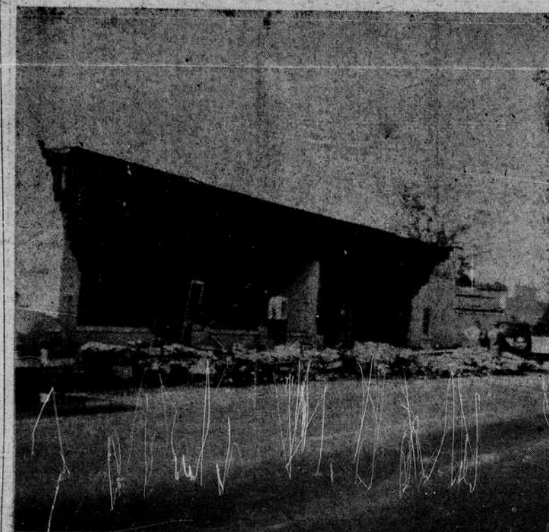
DAMAGE—The front of the Shallotte Motor Sales building at Shallotte was badly damaged by the storm, which caused considerable other destruction to buildings in that town.—(Graham Fore Photo.)
