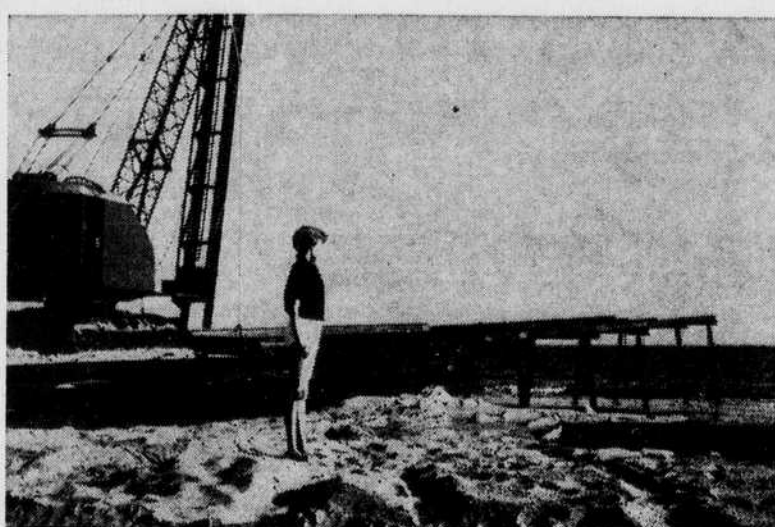
BUILDING—Miss Joan Bryant is shown as she surveys the first stages of construction of the steel fishing pier at Yaupon Village. Speedy progress is expected in completion of this project.—(Art Newton Photo.)
