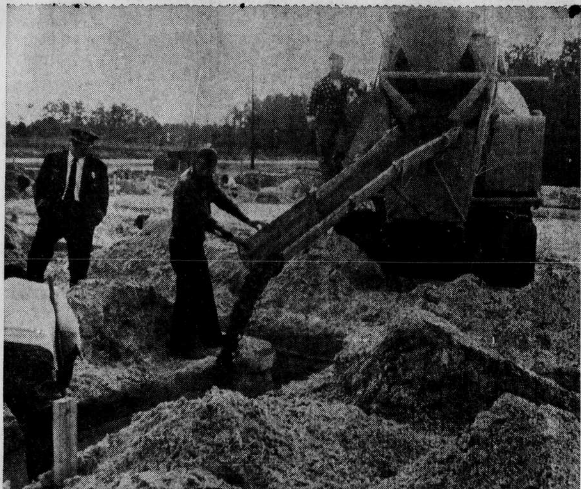
ACTIVITY—Construction began last week on the new National Guard Armory at Shallotte, and in the above photo Shallotte Chief of Police Leon Galloway appears to be an interested observer as two workmen pour a section of the foundation for the new building.
