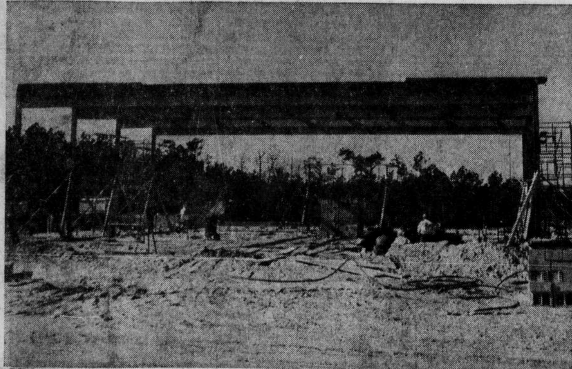
CONSTRUCTION—Steel girders for the roof of the Shallotte Army were going up when this picture was taken several days ago. Although bad weather for the past few days have hampered construction operations, good progress is being made.
