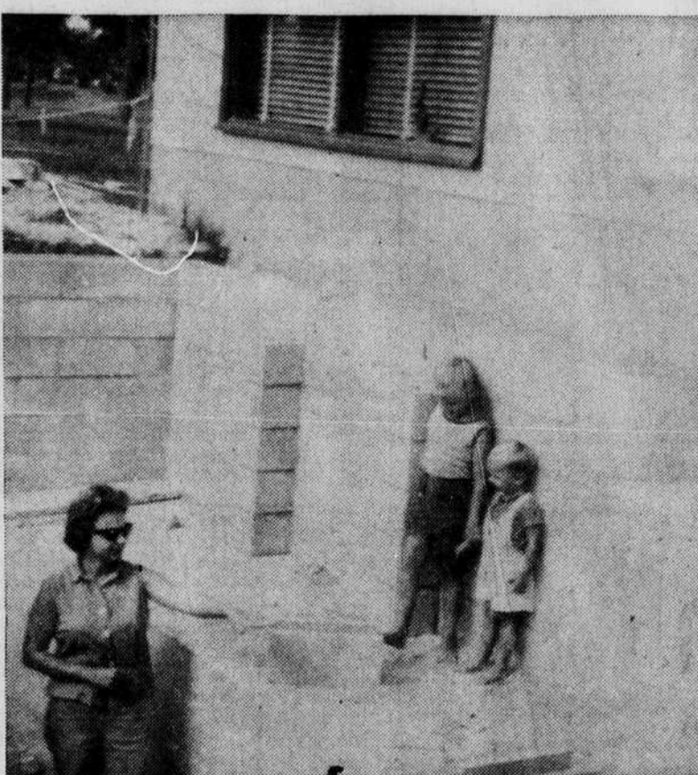
REFUGE—Mrs. Leigh Tomlinson is shown here standing on the floor of the fallout shelter being constructed at the Tomlinson home in Deepwater Heights. Standing by on the sleeping shelf are daughter Mary and son Johnny.
