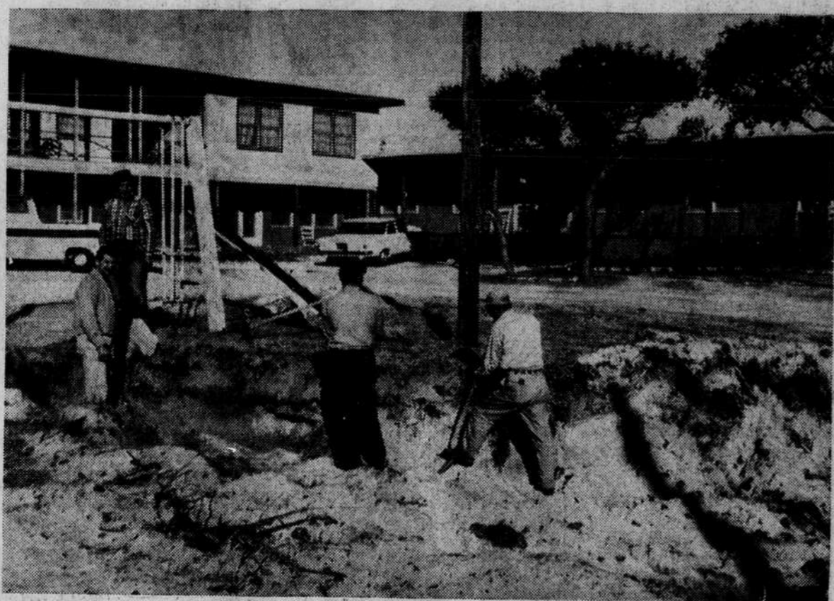
PIONEER —C. E. Murphy and three of his men are shown here shaping the excavation of the freshwater swimming pool which he is building in front of his Oceanfront Motel at Yaupon Beach. He expects to have it ready for use before next summer. It will be the first swimming pool for any of the Brunswick County motels.—(Walker Photo.)
