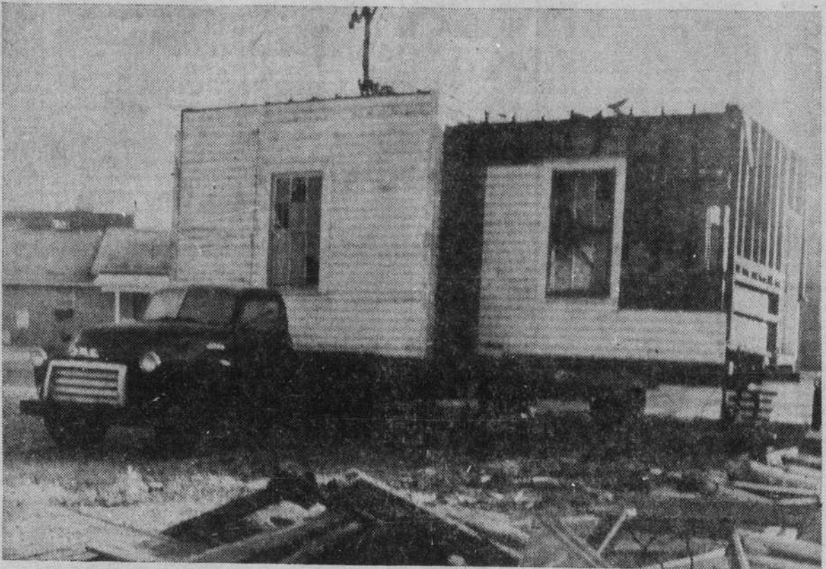
MOVING—The two-story home standing on the lot where the new Waccamaw Bank & Trust Co. office will be constructed has been torn down to a single story, and that has been loaded on a truck and moved to a new location near Dasher Memorial Hospital. This was a scene of the moving operation taken early today. (Staff Photo by Allen)
