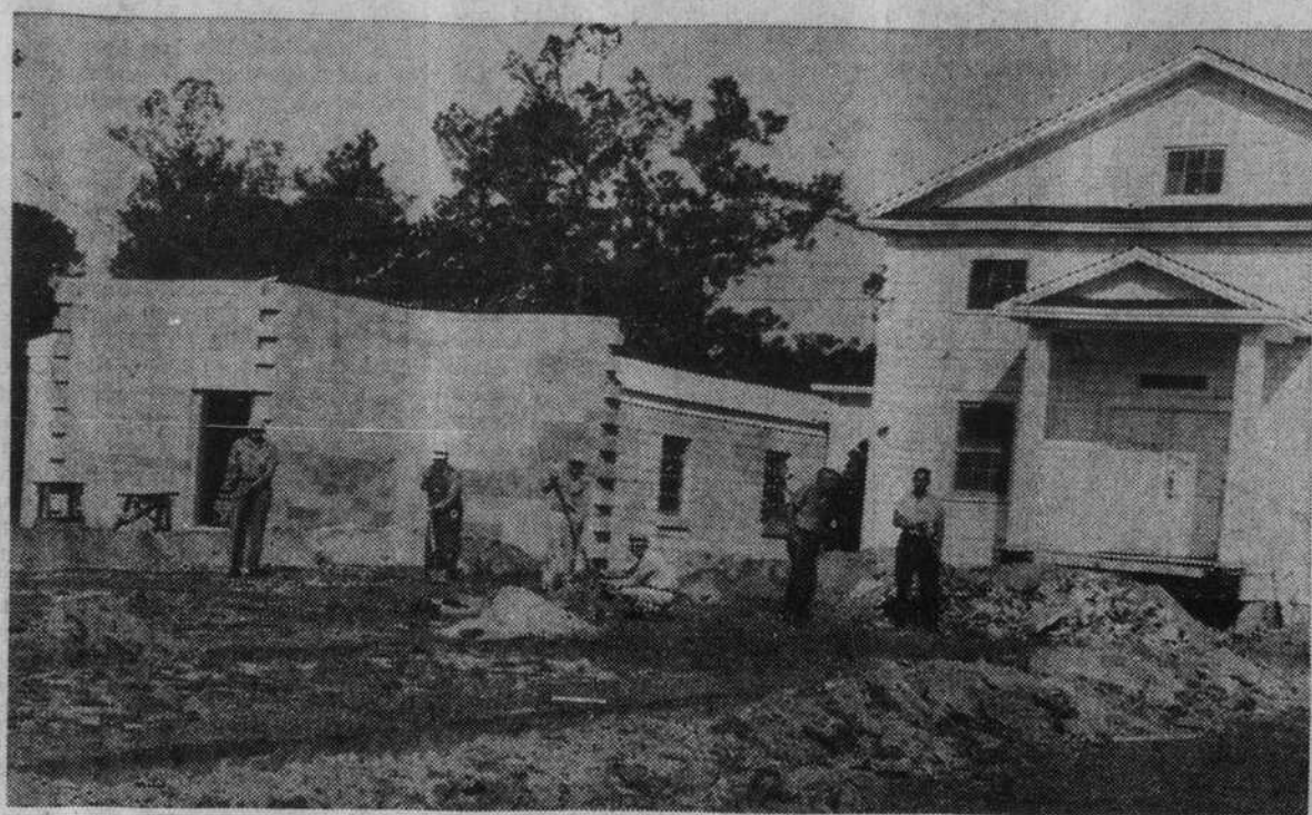
FOUNDATION—Work has begun on the foundation for the sanctuary of the First Baptist Church in Shalotte, formerly Chapel Hill Baptist Church. Ground breaking ceremonies were observed Monday. (Staff Photo by Allen)
