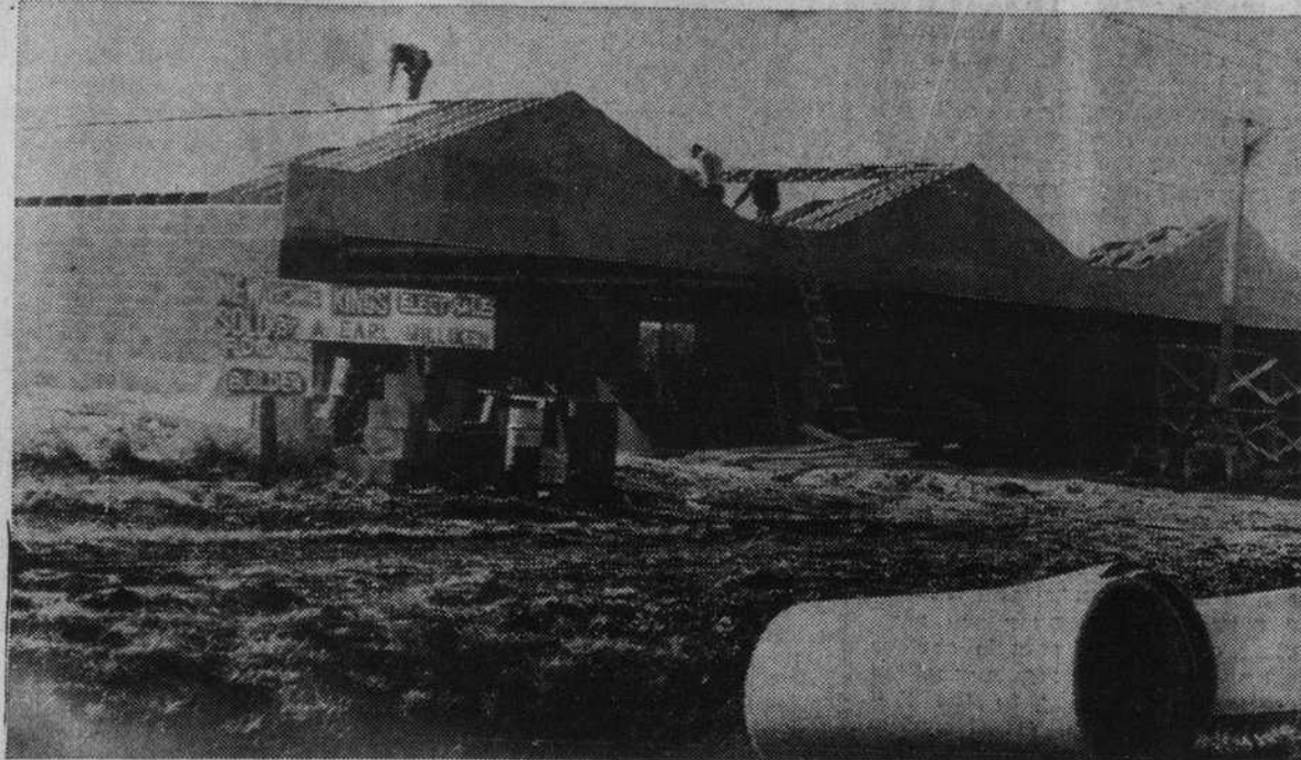
CONSTRUCTION —This big new building is being erected as the future site of a furniture store. It is situated on U. S. 17 on the outskirts of Shallotte. It has a 100-foot frontage and is 80-feet in depth. The owner is Eli Kravitz and the contractor is Floyd King. (Staff Photo by Allen)
