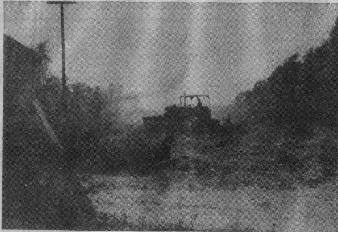
CLEARING —State Highway forces were busy last week clearing the right of way for the extension of West Street to the site of the Southport Small Boat Basin for which contracts will be opened next Tuesday. (Staff Photo by Allen)
