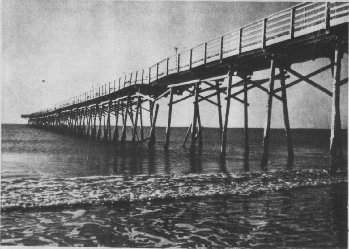
Where Boat Hit The Pier
