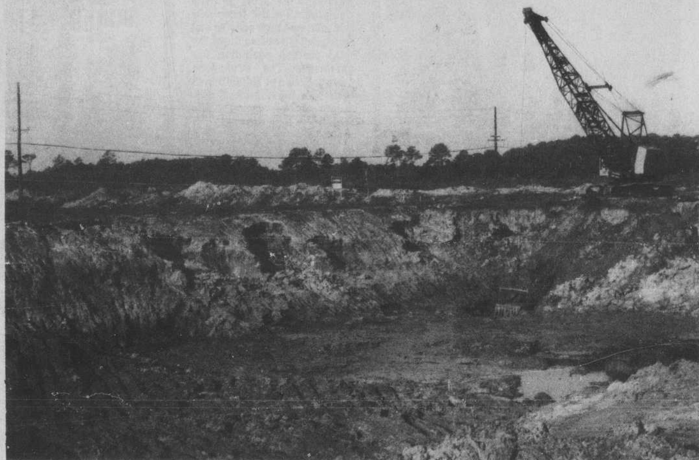
Good progress is being made by workmen in cutting a segment of the discharge canal from the CP&L plant near Southport. They have made the cut at Highway 87-133 in preparation for the construction of a bridge. When this project has
