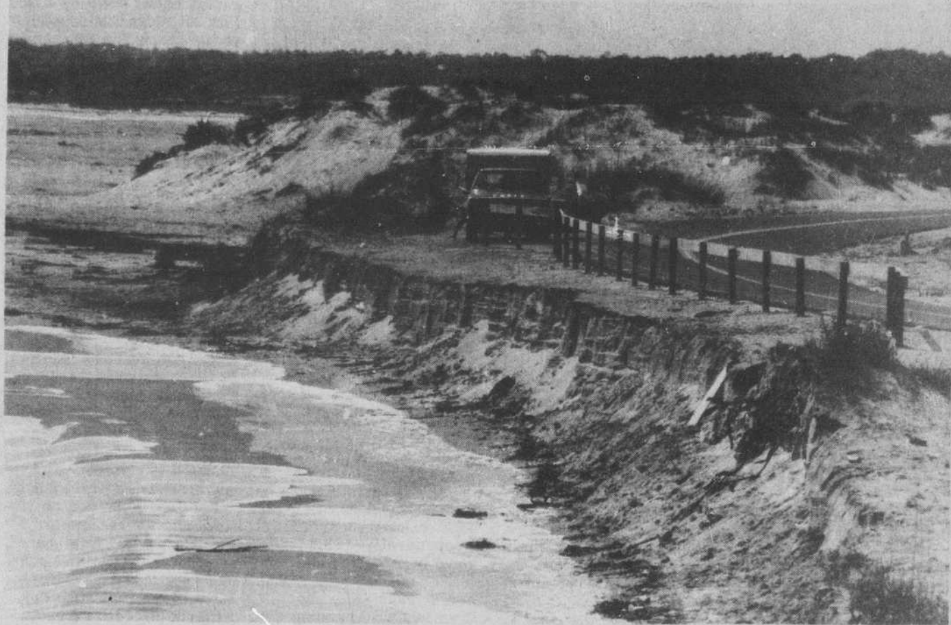
EROSION ON LONG BEACH near Lockwood Folly Inlet slowed during the past week but still threatens the state-maintained road through the King's Lynn section. A series of groins on the
