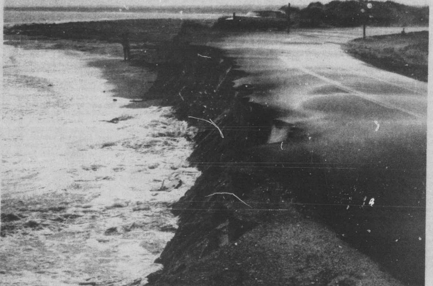
EROSION OF LONG BEACH near Lockwood Folly Inlet was swift and sure Tuesday afternoon as high tides and strong winds undermined the state-maintained highway. At a Friday night public hearing held here, a Corps of Engineers recommendation to proceed with hurricane
