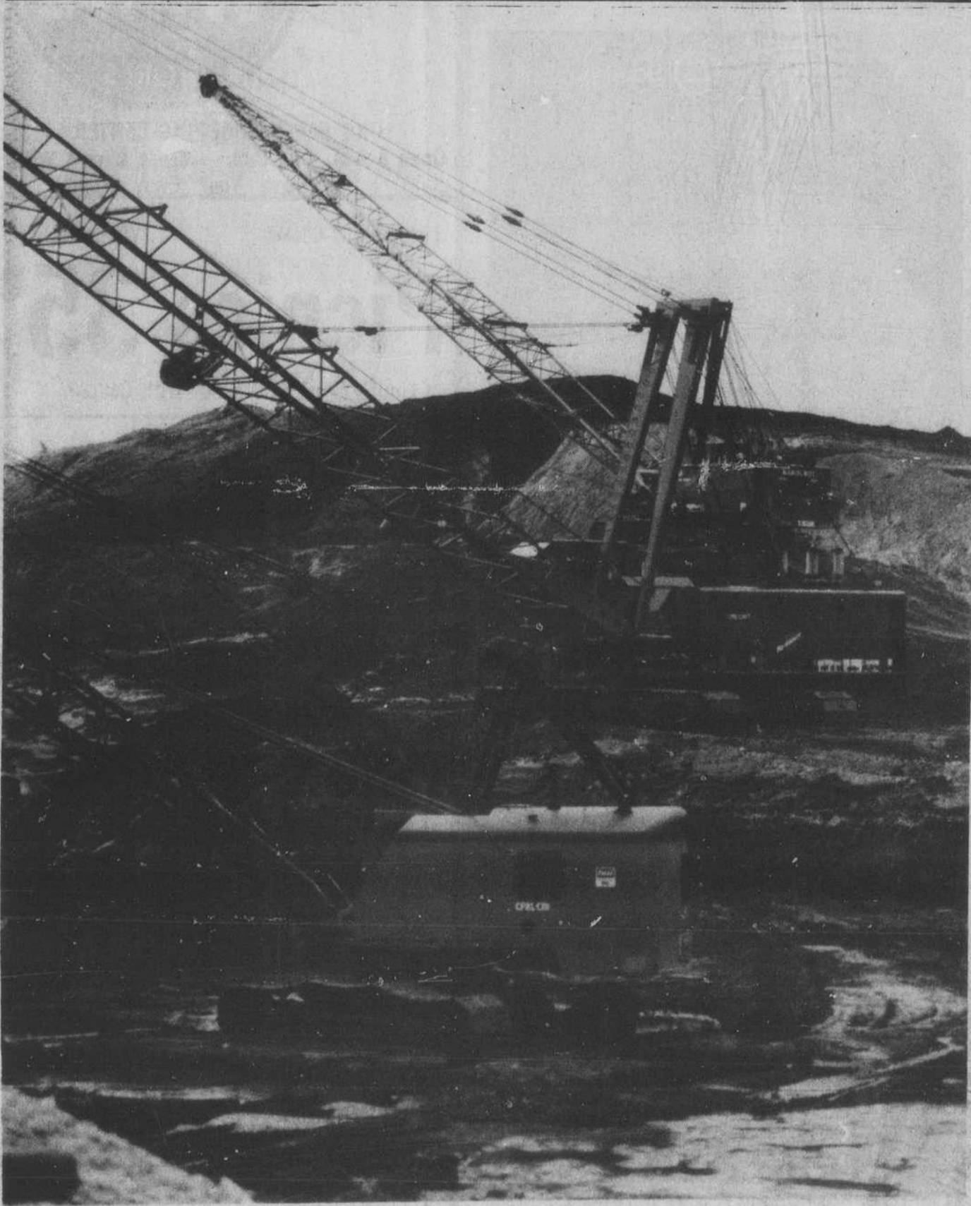
DIGGING OF THE CANAL for Carolina Power and Light Company continues along NC 211 near Southport. This week, the dirt barricade blocking water from underneath the bridge was removed by three draglines, the smaller equipment
