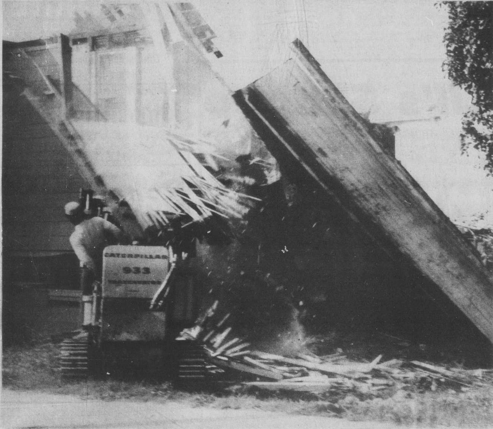
BAILING OUT as the old Capt. James B. Church home comes tumbling down is machine operator James McLean. The old Southport landmark, located at the corner of Moore
