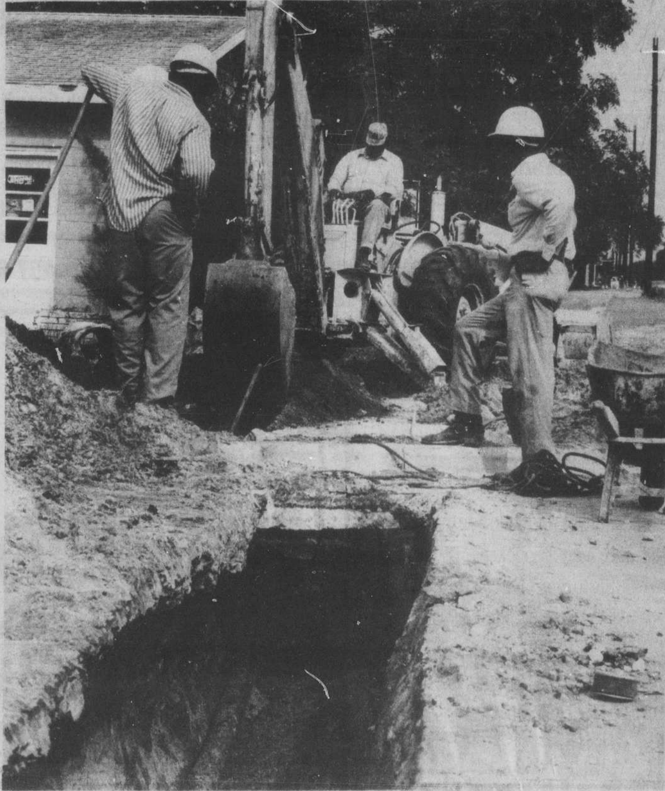
WORK CONTINUES on the laying of telephone cables along the west side of Howe Street. Southern Bell is financing the $65,000 project,
