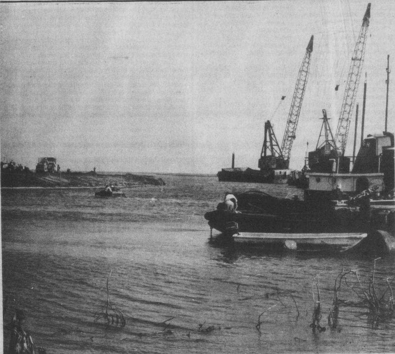
CONSTRUCTION of the CP&L drainage canal is progressing more rapidly than many would expect. Not only has the canal been dug near Highways 211 and 87, but dredges have made their way inland as much as a mile from the Intracoastal Waterway. Here, equipment works
