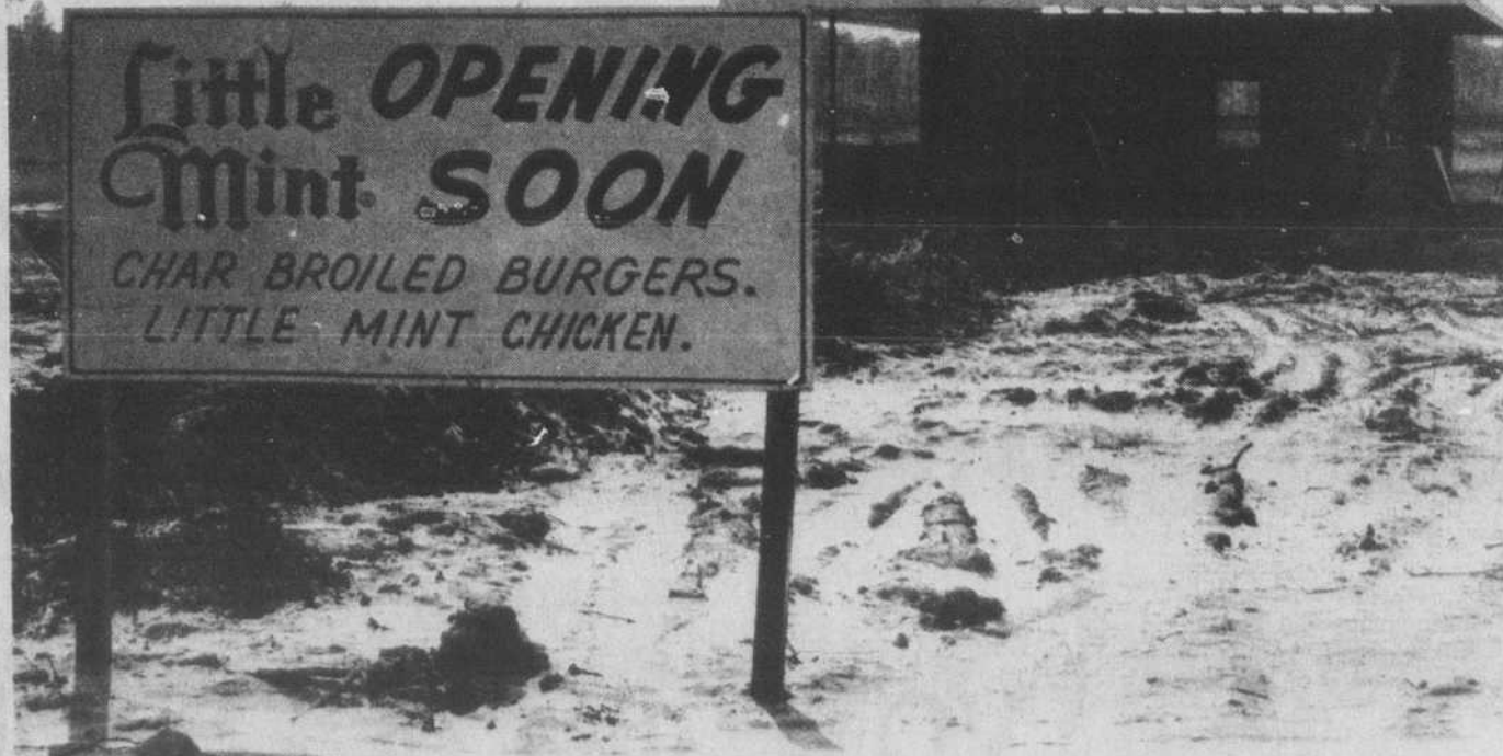
THE LITTLE MINT chain of hamburger and chicken drive-ins is constructing a facility near Southport at the intersection on NC 211 and 87. The chain has several other modern operations in
