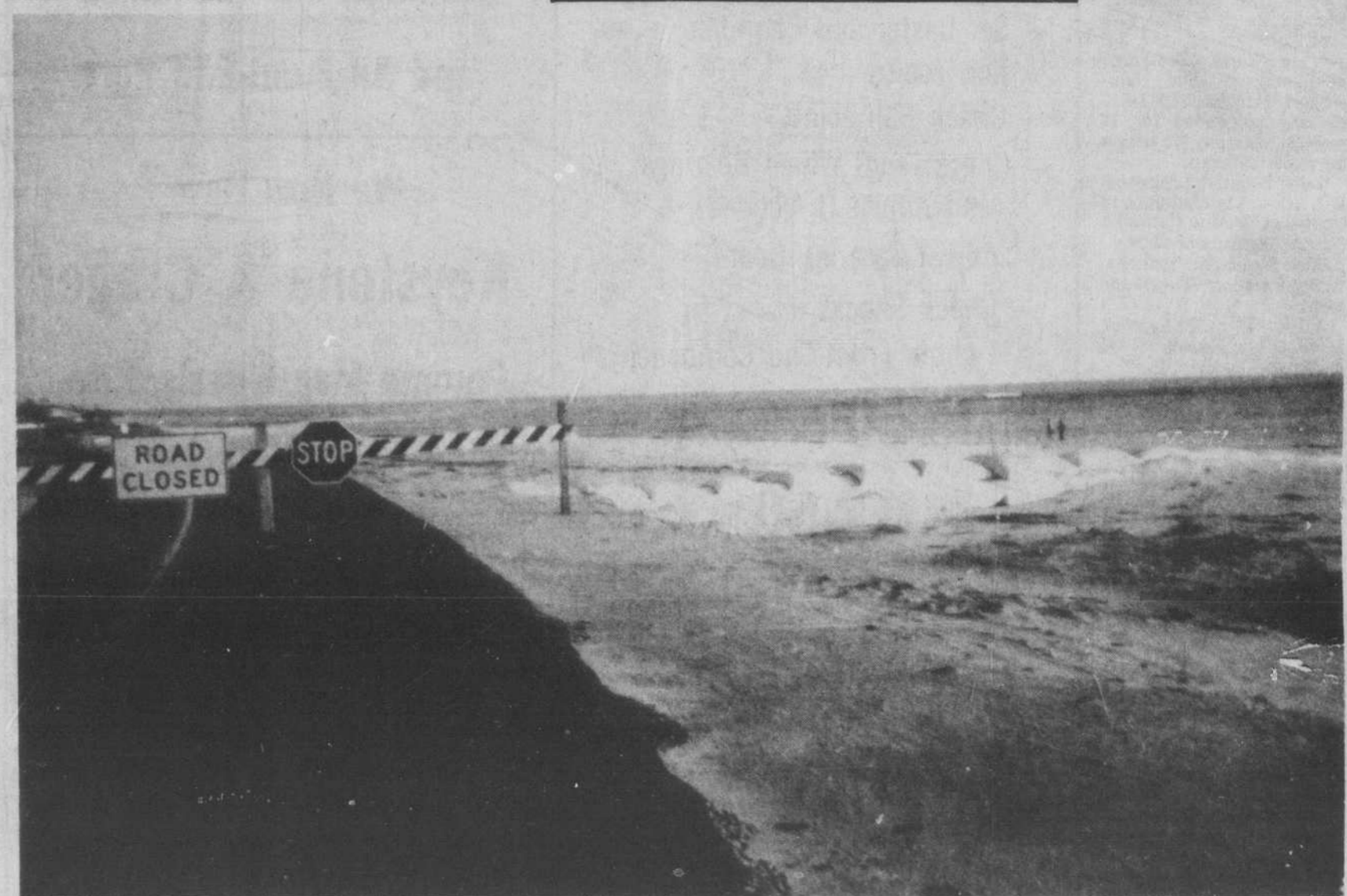
SAND-FILLED BAGS, used successfully at Holden Beach to stem the tide of erosion, are being employed at Long Beach near Lockwood Folly Inlet. The highway was closed last summer after wind and water eroded the pavement. The sandbags, known as groins, are placed perpendicular to the
