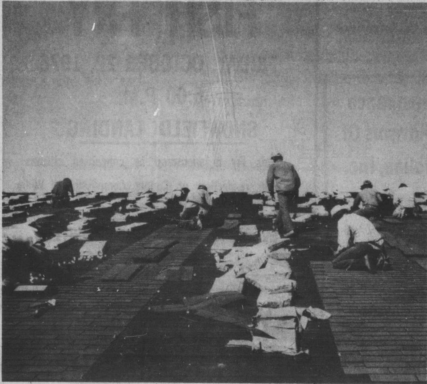
PATCHING THE ROOFS at high schools in Brunswick County is a project underway now, sponsored by the county Board of Education. The roofs at the three high schools have leaked since the buildings were occupied four years ago, and
