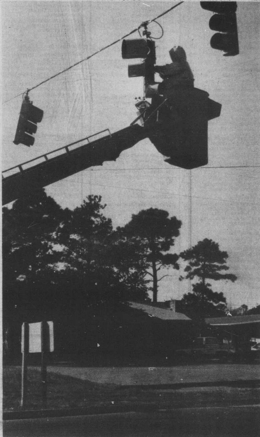
NEW TRAFFIC SIGNALS have been installed at the intersection of NC 211 and 87 at Sawdust Trail, completing the project that also includes turning lanes at the busy junction. The lights presently are flashing yellow, giving motorists a chance to become accustomed to the signals before switching to red and green.
