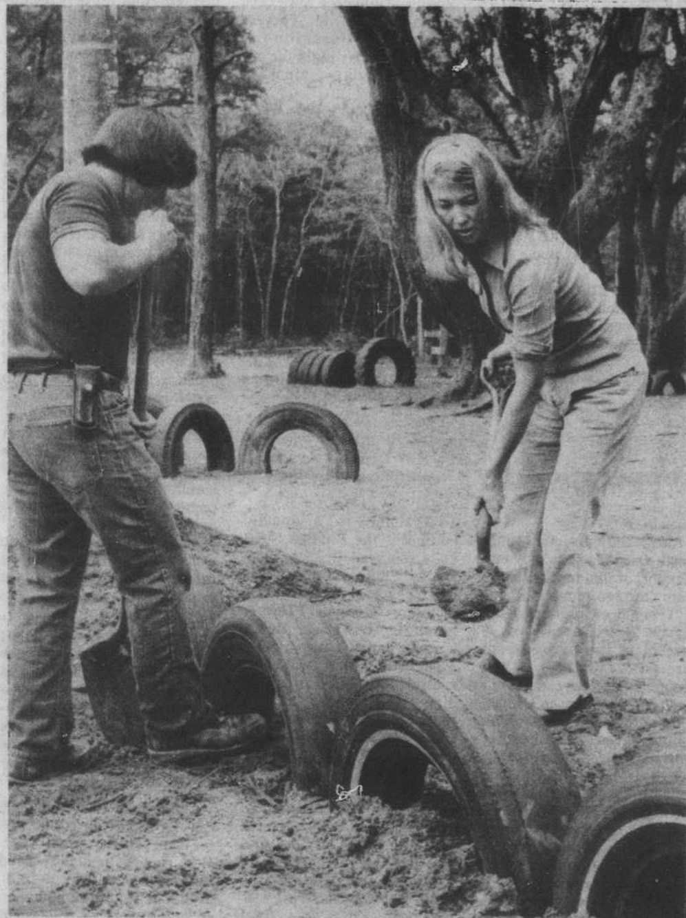
WORK IS PROGRESSING, but slowly, on a playground for children at Southport Primary School because volunteer labor has been in short supply. But two faithful workers, Faith Birkhead and Bob Phillips, were on hand Saturday morning to lend their help to the project. Ms. Birkhead said anyone interested in helping should be at the site behind the primary school Saturday morning at 10 o'clock.
