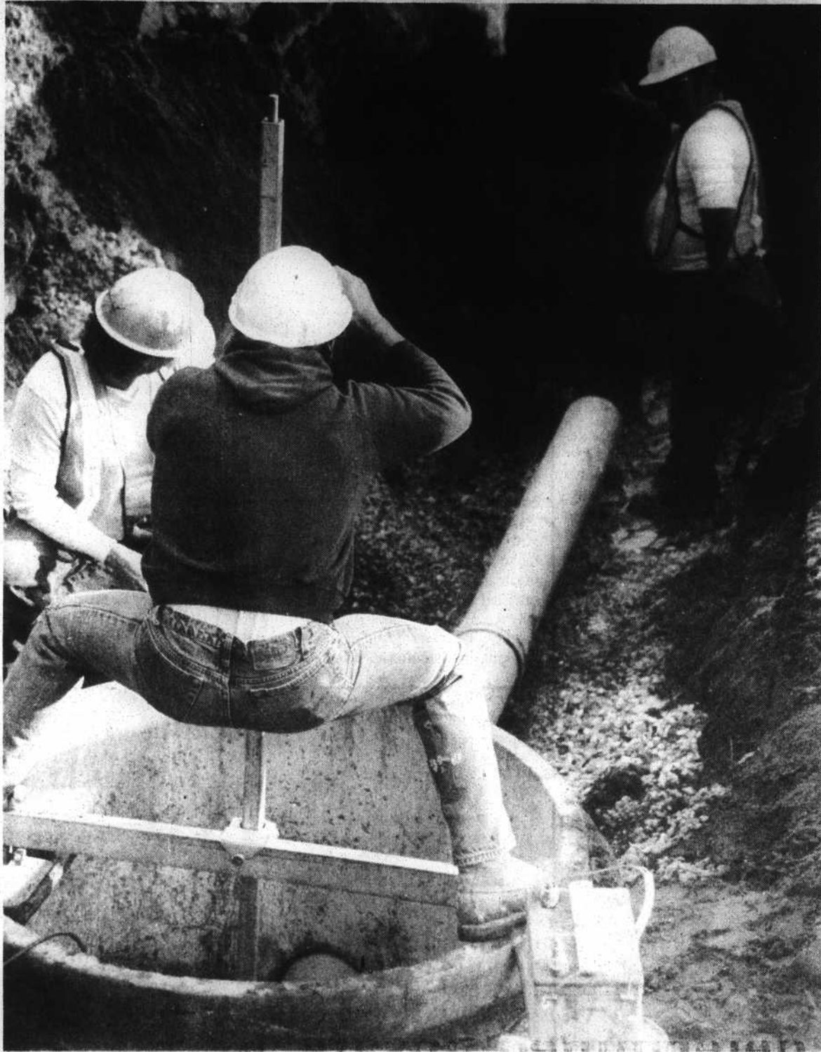
Work continued this week on the reconstruction of Cape Harbor Drive in Southport. The street is to be totally rebuilt. Additionally, water and sewer lines beneath the street are to be replaced. City officials
