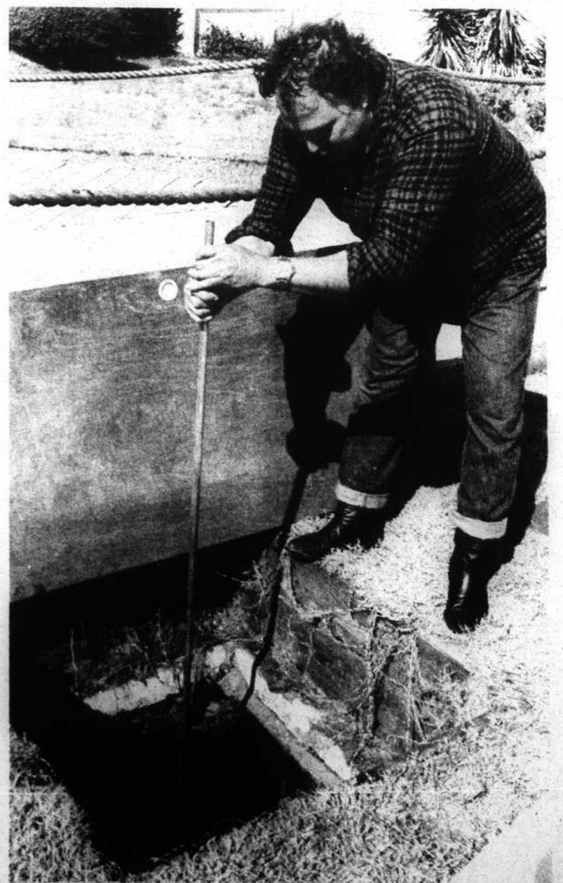
Tom Dean prods the bottom of an old faulty septic tank constructed of cinderblock on his newly purchased property, the Blue Water Point Marina.
