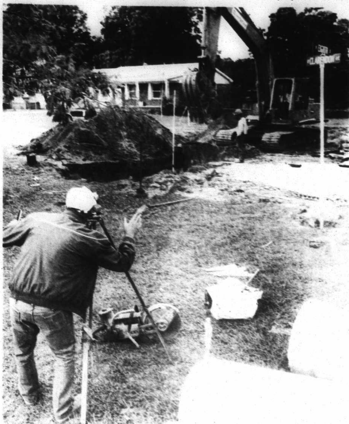
Work was underway this week on the drainage projects on West 8th Street and at the corner of Lord and West 9th streets. The work is expected to be completed within 60 days.
