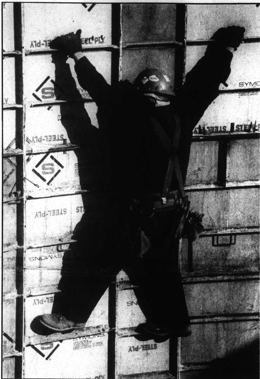
Rebarco employee Phillip Hair this week prepared to take down the forms inside the Yaupon Beach sewage treatment plant on Fish Factory Road. Construction of the plant is running on schedule and should be completed in August. An estimated 42 million gallons of water will be treated annually.
