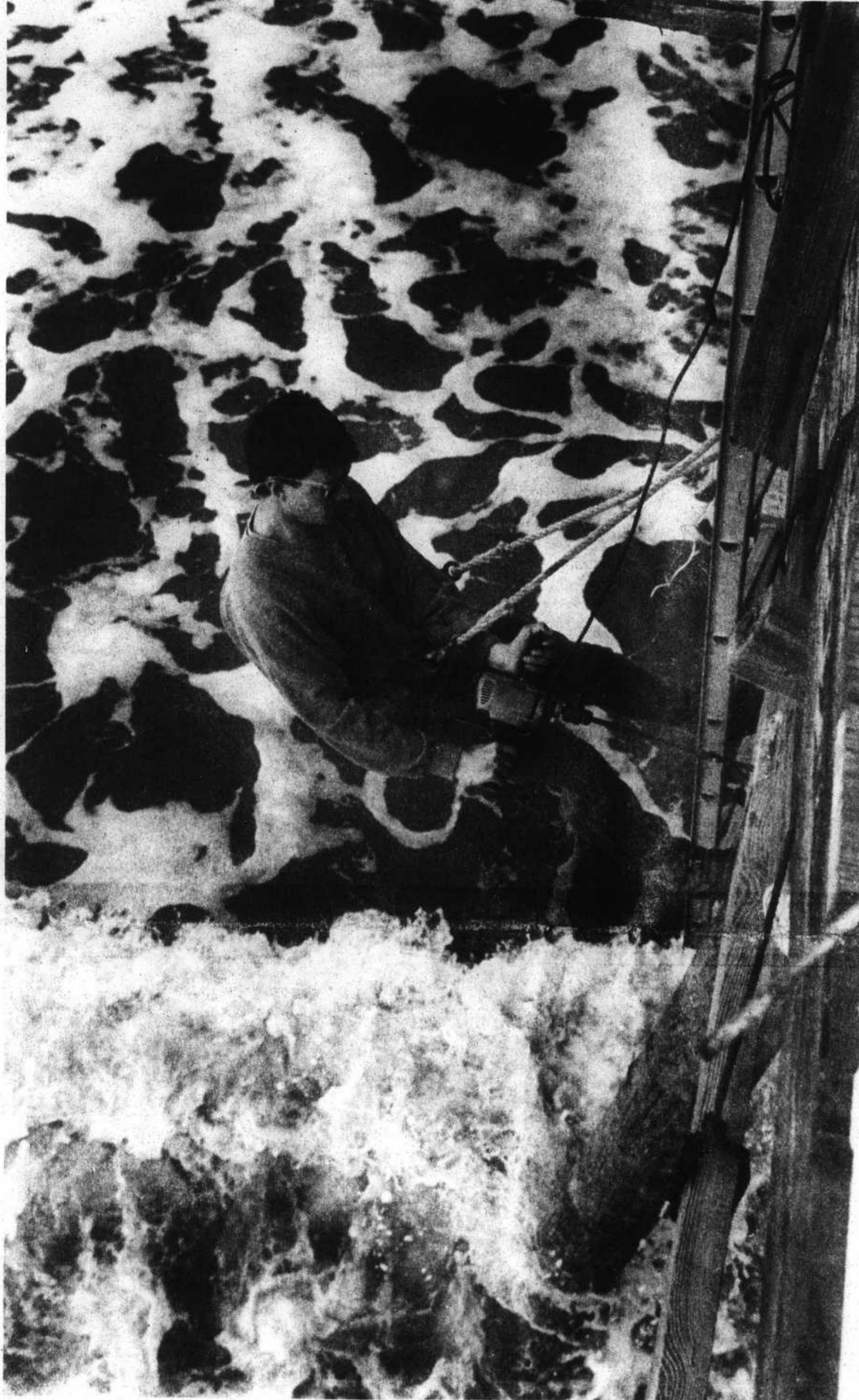
Long Beach surf crashes shoreward under a workman sinking a bolt hole in new piling at Ocean Crest Pier. Work continues this week on replacement of pilings and repair of pier decking.
