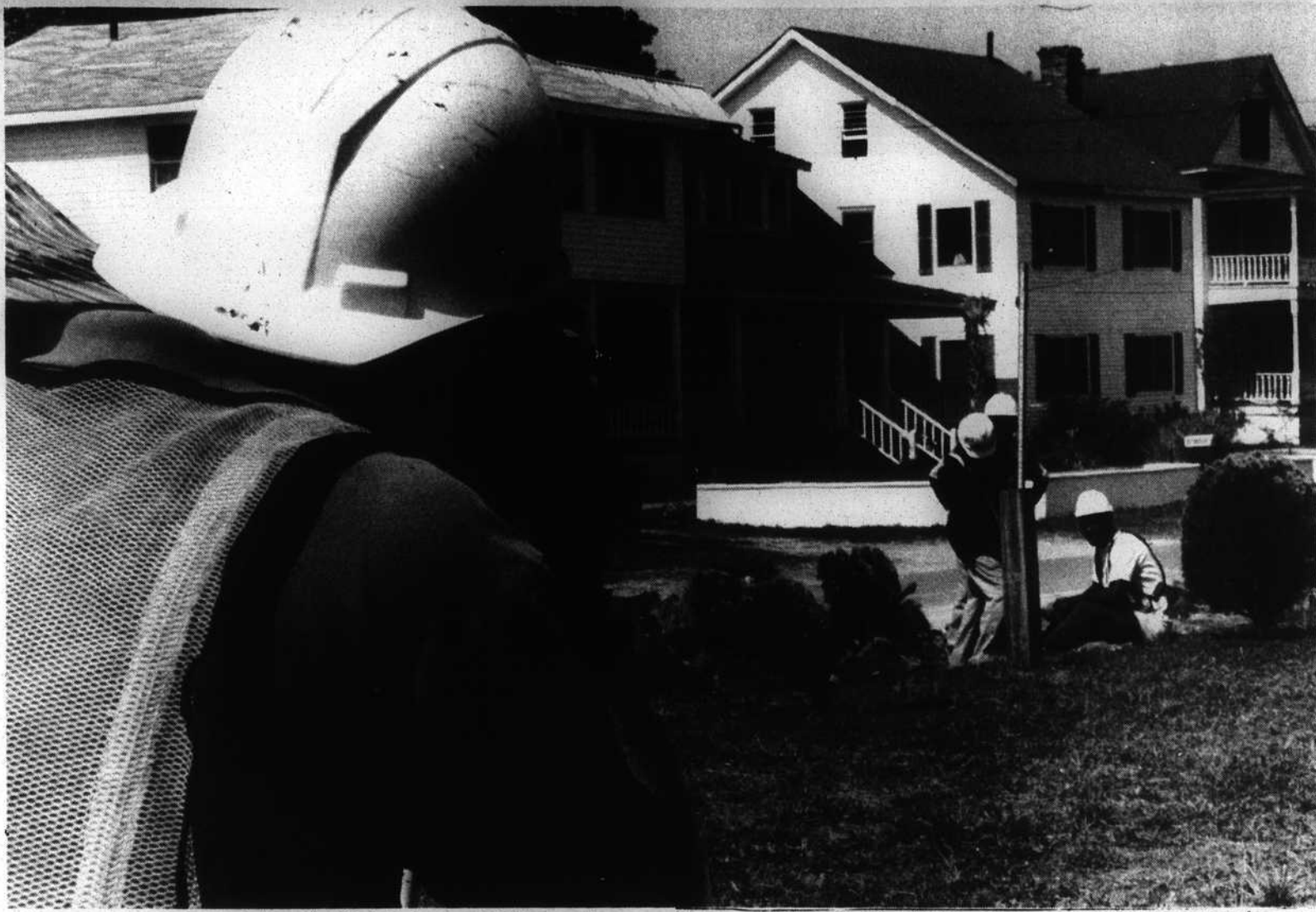
Southport city workers this week officially began the Riverwalk project by starting to lay nearly 700 feet of sidewalk along Bay Street from the pilot's tower to Port Charlie's Restaurant. City officials hope
