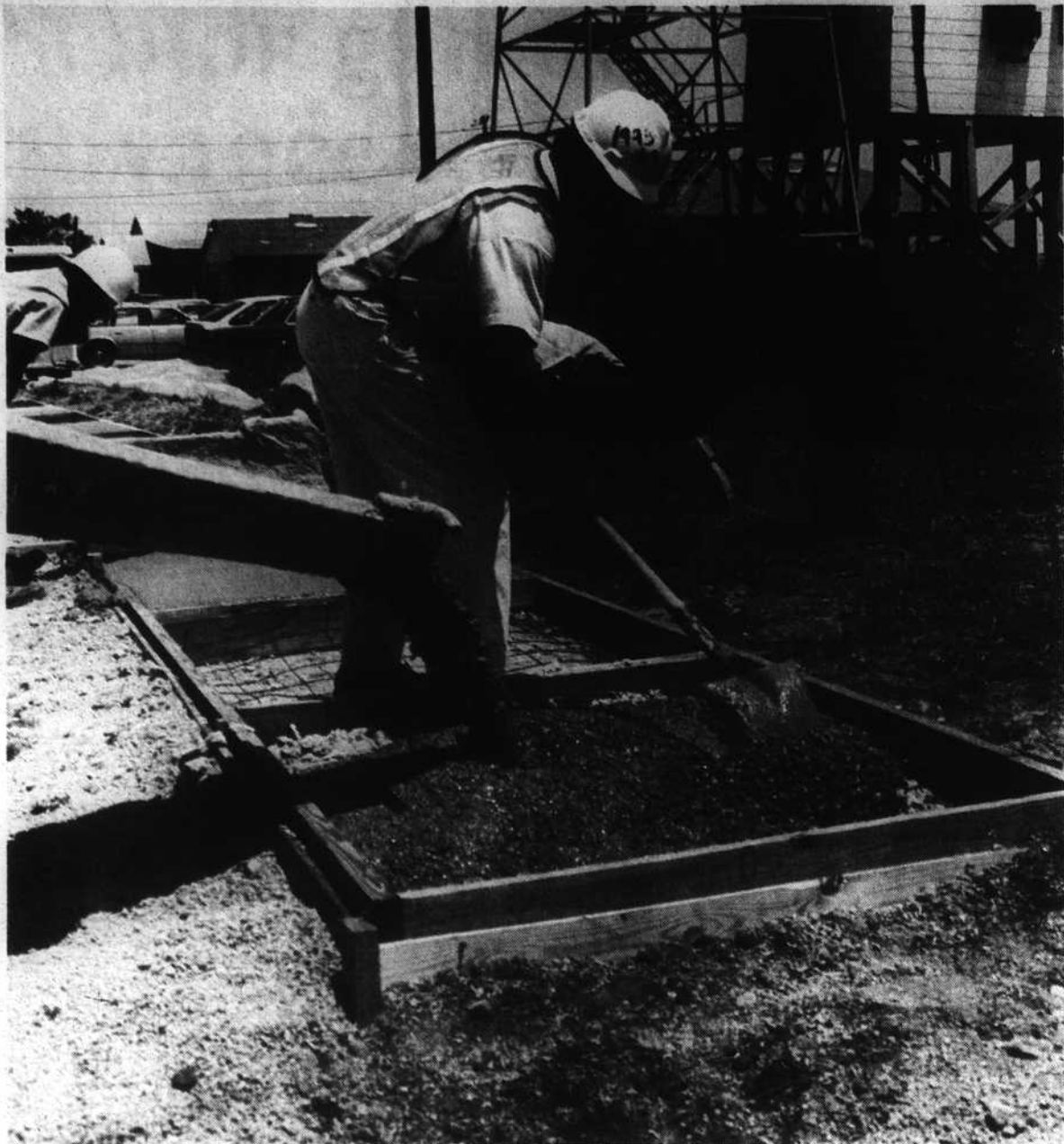
Kenny Price spreads concrete for the new River-tween the pilot tower and Port Charlie's walk segment which city workers are installing between the pilot tower and Port Charlie's Restaurant.
