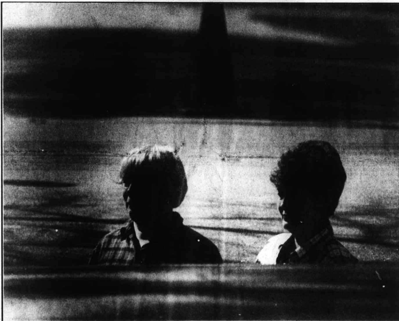
This is what a motorist would have seen Saturday afternoon as Boiling Spring Lakes residents Julie Brown and Carol Gallagher inspected a sinkhole that opened up earlier in the day on Berryhill Road.
