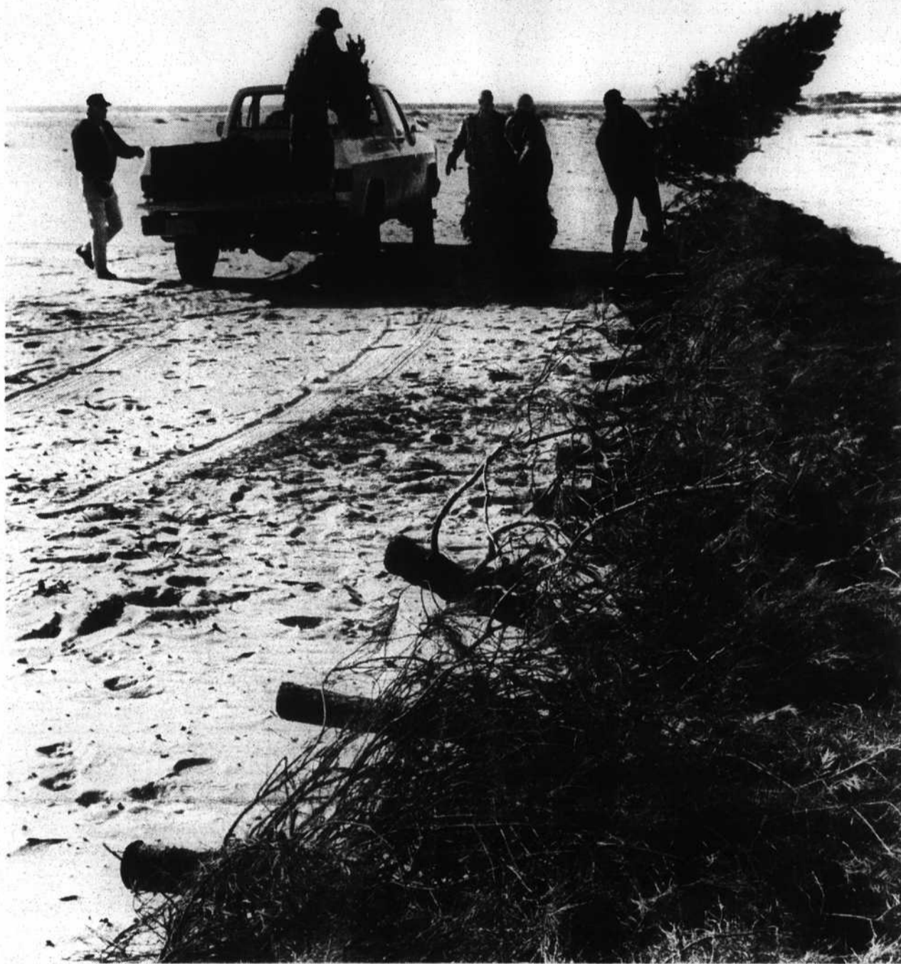
Photo by Jim Harper Brunswick County extension agent Bruce Williams, volunteers and Long Beach town employees this week constructed sand fences with discarded Christmas trees near the western point of the Long Beach strand. Three 50-foot sections of fence were erected; Williams will return to the same location in March to plant beachgrass. The point of the experiment is to show beachfront property owners that they can help minimize erosion.
