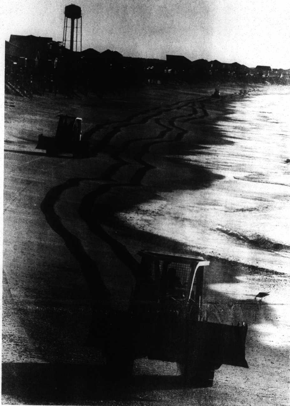
Mac Construction earth-moving equipment operators began pushing sand at Long Beach Monday in an effort to restore dunes damaged in a series of recent winter storms.
