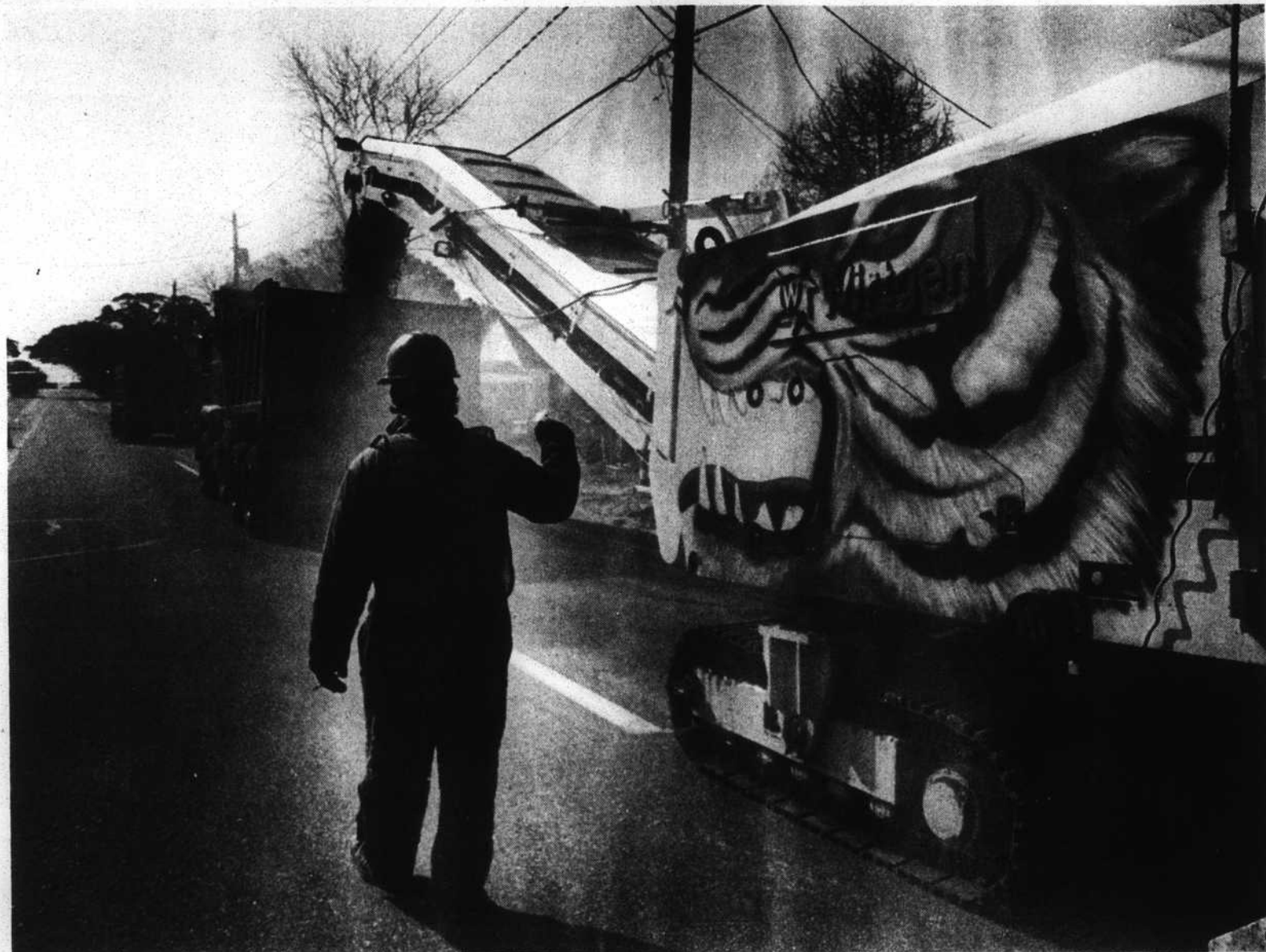
Crews under contract to the state Department of Transportation have been at work these last two weeks preparing Southport's Howe Street for resurfacing. This vehicle is a milling machine that textures the existing road surface in preparation to accept new asphalt. The Howe Street work is expected to continue for two to three weeks.
