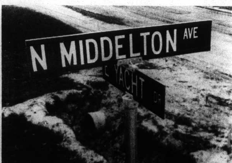
Work on the Yacht Drive paving project also involves construction of drainage swales and ditching.
