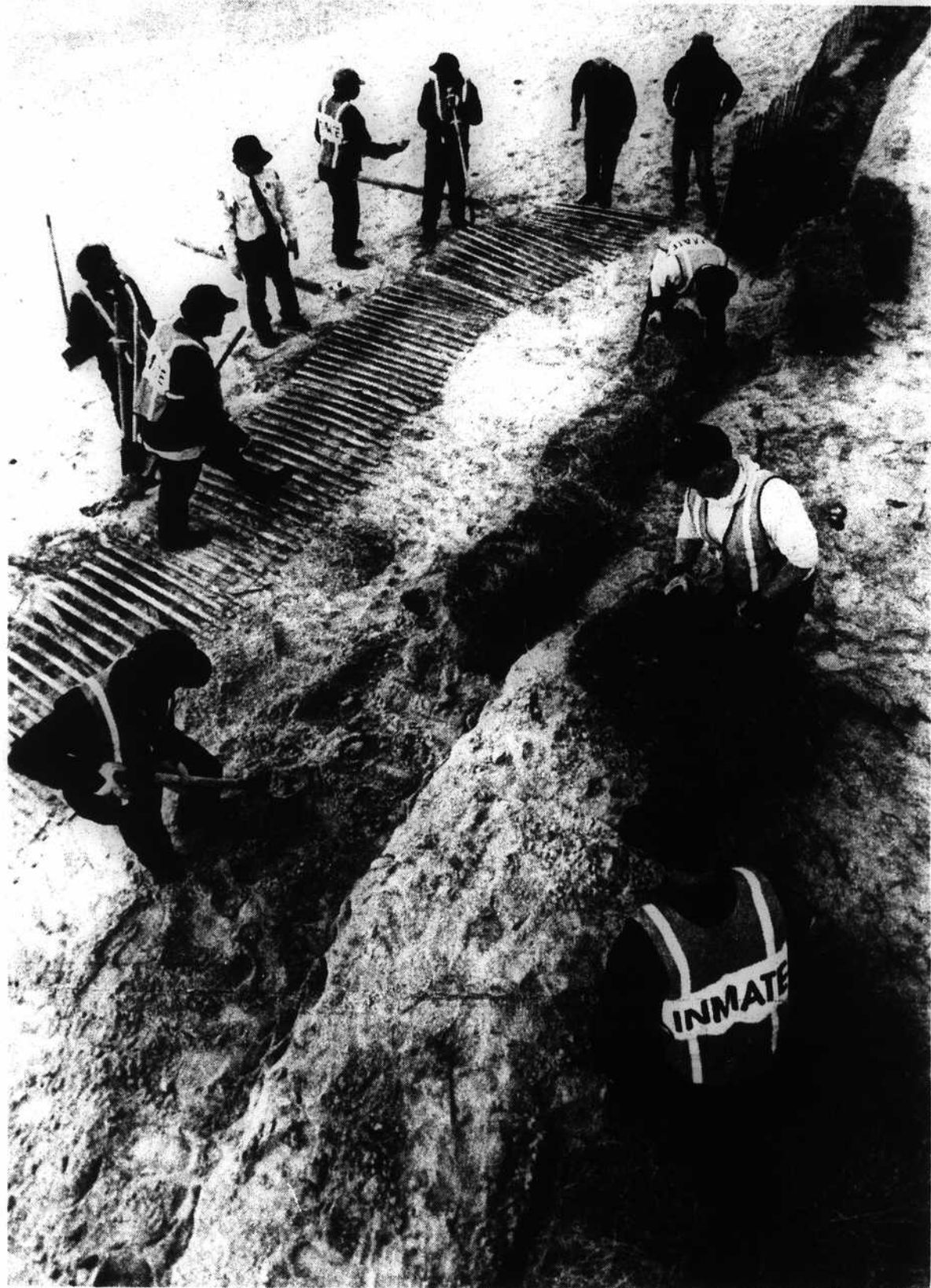
Inmates from the New Hanover state correctional unit are at work again this week on a number of Caswell Beach public works projects. Besides repairing sand fence along the beachfront they will also mulch roadside plantings, clean up the beach access parking lot and work around Town Hall.
