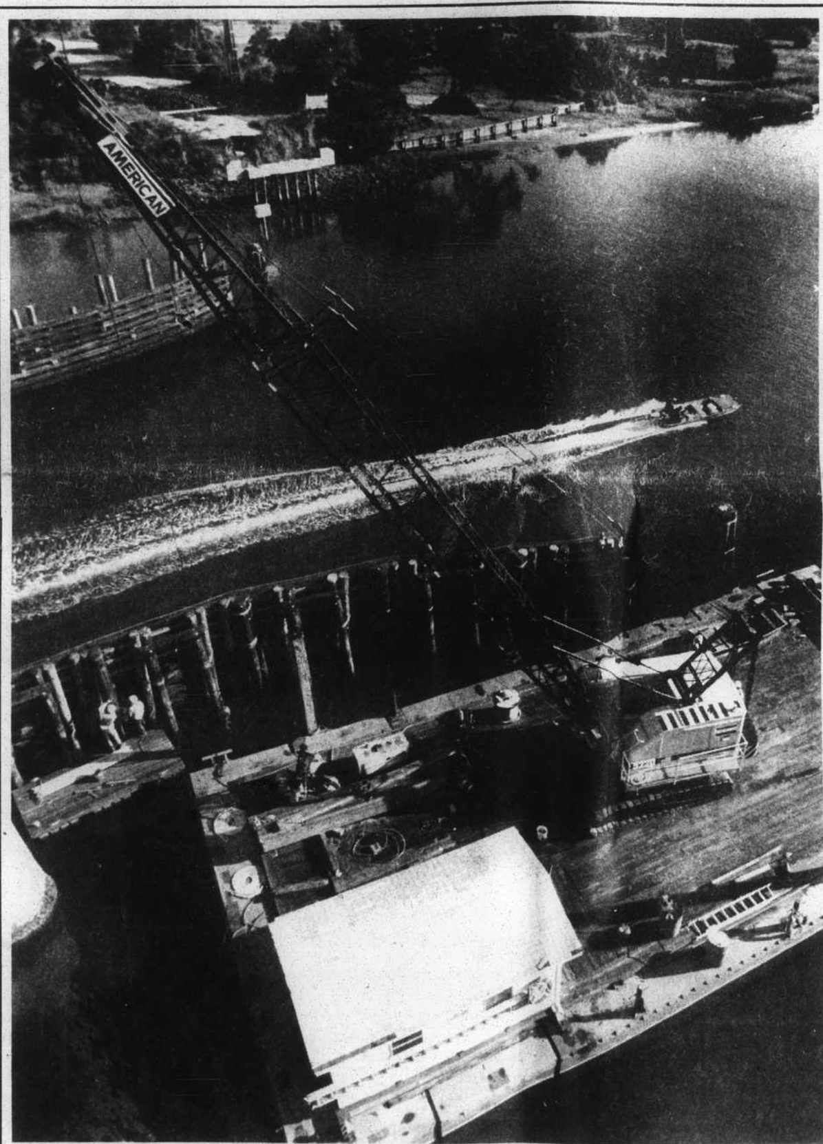
Repair work continues this week on the approach wings leading underneath the Oak Island bridge. Periodic maintenance is required on the wooden structures which ensure that watercraft passing beneath the span do not touch structural parts of the bridge.
