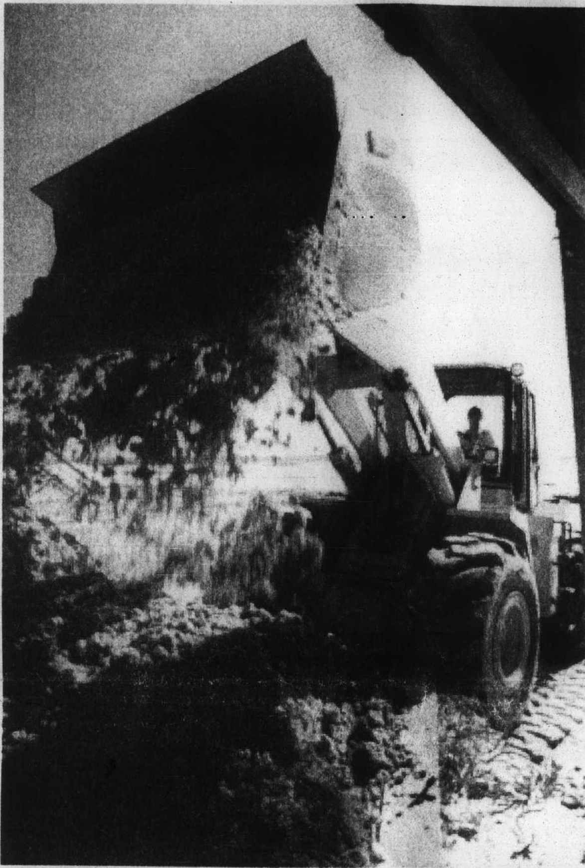
Dune repair has been a critical part of town response to a series of nor'easters which struck Oak Island and the Brunswick County shoreline last week. The effort at Long Beach has included use of the town's wheel loader. Long Beach crews are now doing beachfront maintenance work the town previously had to hire contractors to do.
